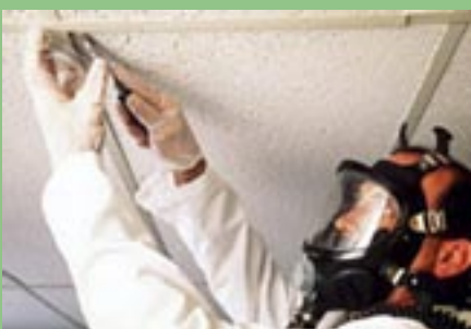
Asbestos fibers can cause significant health problems when inhaled.
